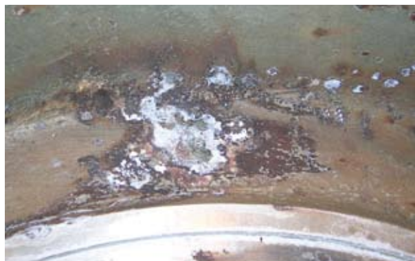
Pitting corrosion attack
